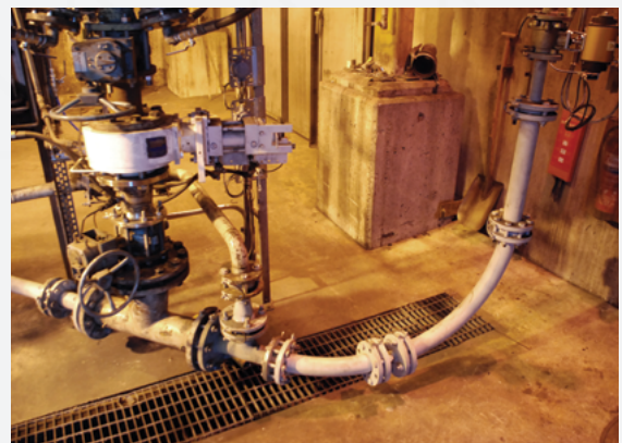
Pneumatic conveying of soot from a blast furnace
