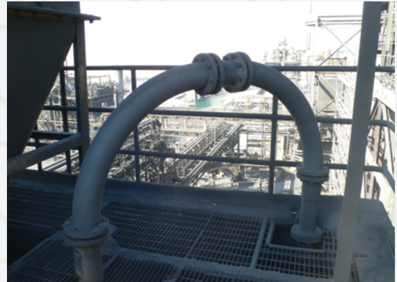
Pneumatic conveying of copper concentrate in a copper smelter
